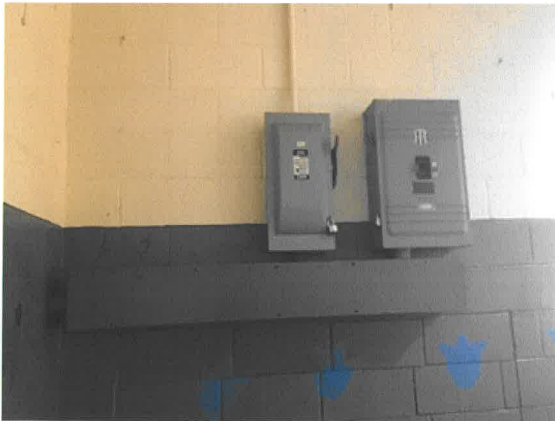
FIGURE 4 EXISTING 100AMP DISCONNECT, RTU SERVICE CIRCUIT BREAKER, AND WIRE TROUGH. THE DISCONNECT IS THE CURRENT SOURCE FOR THE RTU. WIRING IS TO BE REMOVED FROM THIS DISCONNECT UP TO THE RTU.
